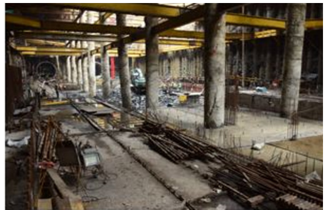
Figure 8: Station construction at 3 major stations Source: Mumbai Metro Rail Corporation Limited; for more details – www.mmrcl.com
